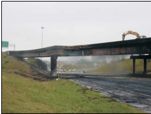
The intense heat of a diesel fuel fire caused this bridge to warp and buckle, closing the highway entirely.
