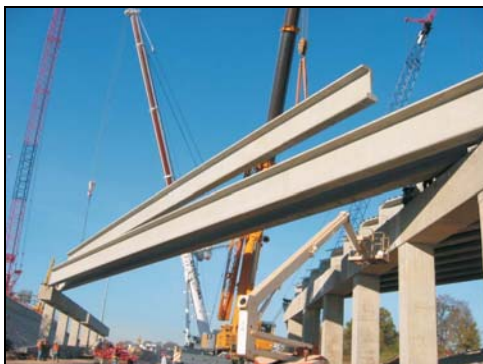
Sherman's high quality pre-stress girders helped get Alabama rolling again in record time.
